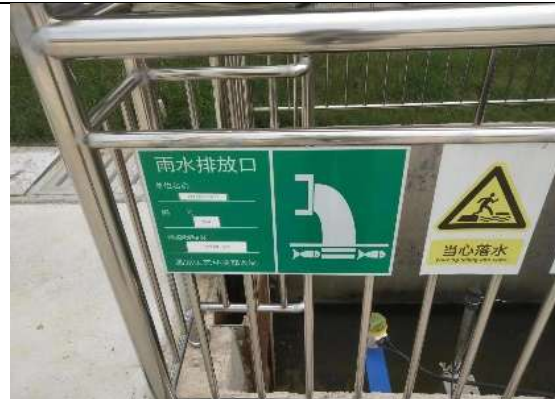
雨水排放口切断闸阀
